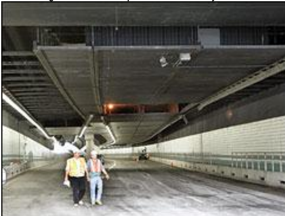
Figure 11: Firefighters inspect a section of ceiling in the Interstate 90 eastbound connector tunnel through Boston that collapsed onto the roadway
